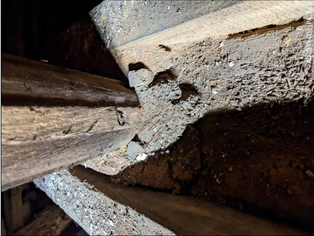
Plate 15 – Truss 8 – North – Remains of original sole plate
