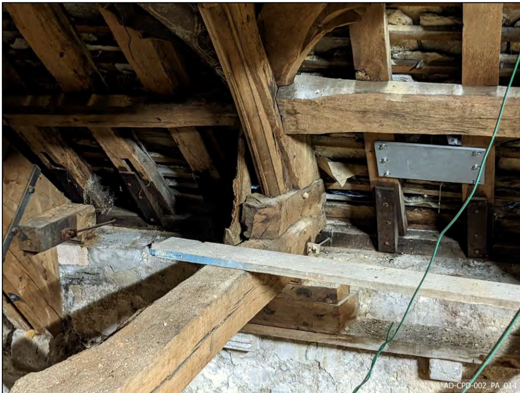
Plate 14 – Truss 2 – South – Alterations to original sole plate
